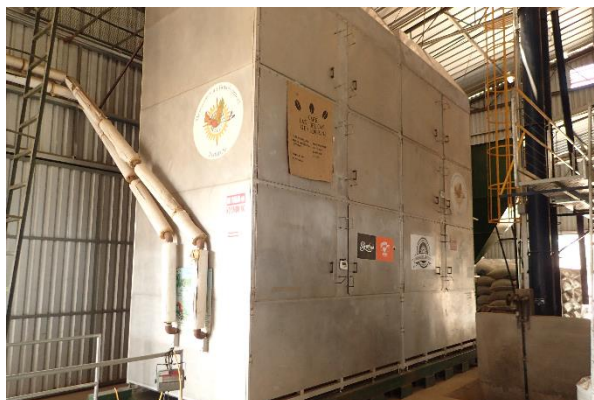
Five more hybrid solar-thermal coffee dryers will be installed this year.
